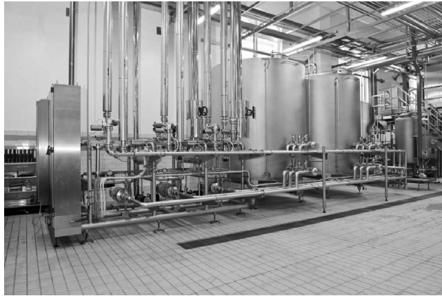
Fig. 7.23 A compact CIP module integrates the tanks for cleaning chemicals, hot and cold water. The system is automated and directly connected to the filler.
