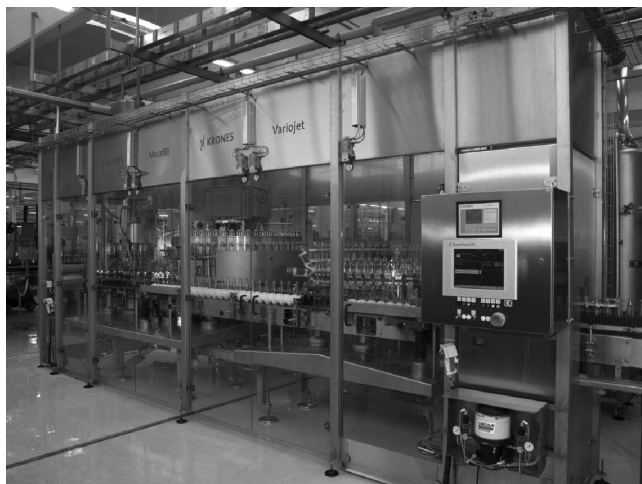
Fig. 7.22 Filler in a cleanroom with hygienic guarding.
